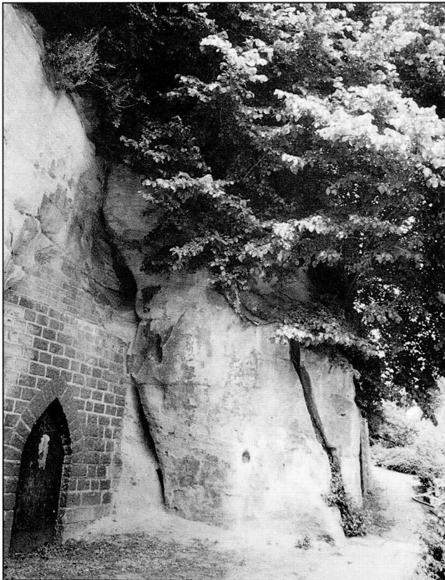
Fig. 4. The widening fissure beneath the unstable sandstone slab beside Castle Road, before the trees were removed and the rock was bolted.
